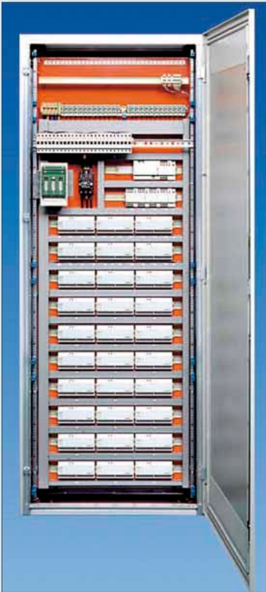
dimmer rack cabinet
