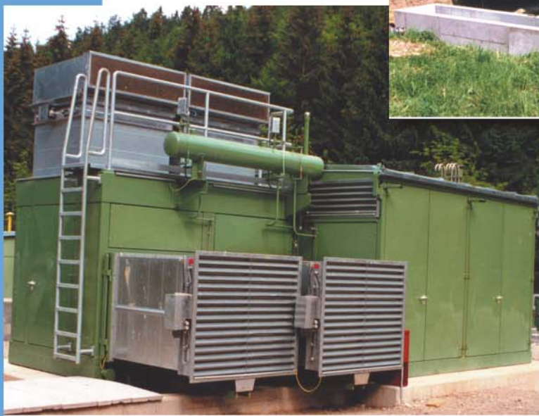
▲ Two VGd 1314 W 2.8 models, supersilent, maximum delivery 74.3 m 3 /min (2770 scfm), suction pressure 7-18 bar (102-261 psi), working pressure 28 bar (406 psi), driven by 108 kW (145 hp) natural gas engine
