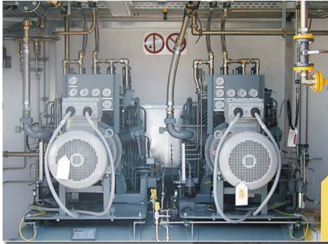
◀ Two CNG compressor units V16G-4411 L 25
